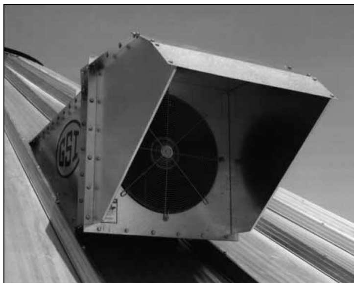
Figure 7B 24" Roof Fan Exhauster with the Rain hood in Place.
